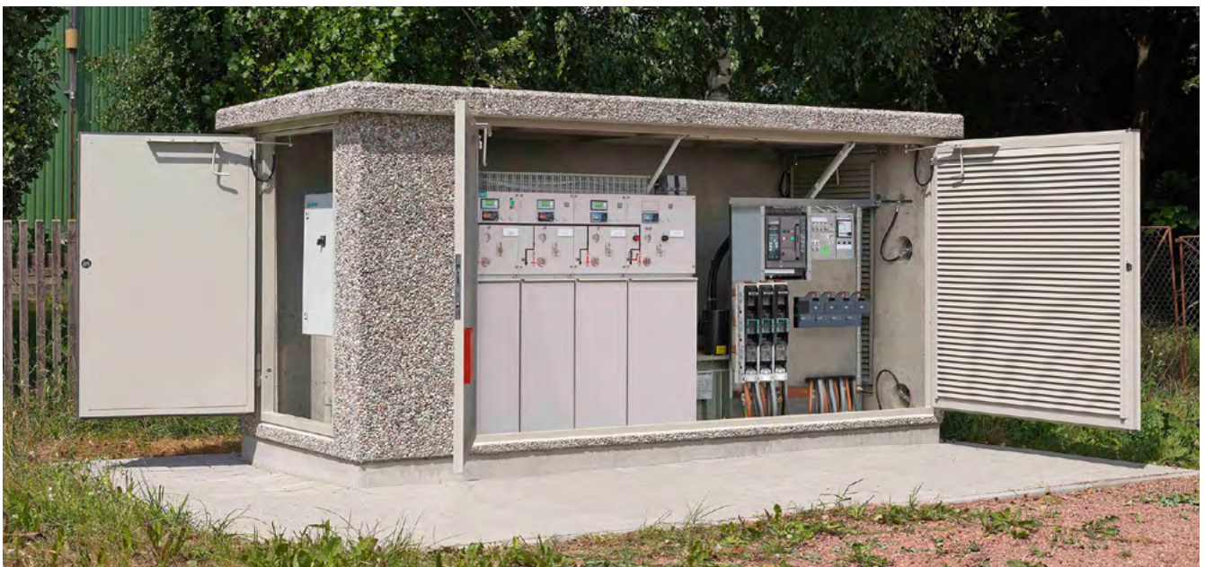
Fig. 2.6-5: Intelligent transformer substation
