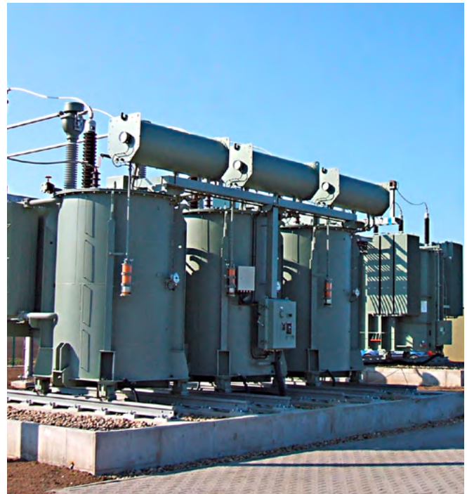
Fig. 4.2-38: Variable shunt reactor
