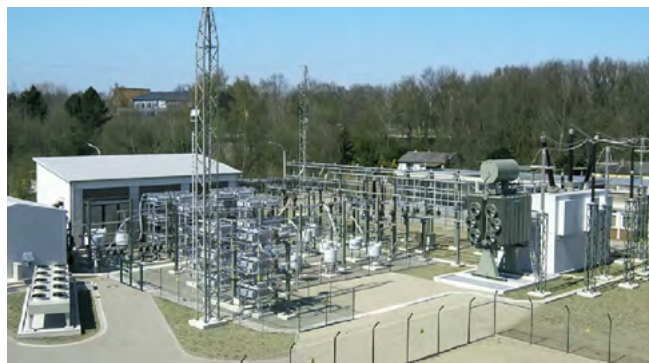
Fig. 2.2-19: Static Var Compensator (SVC) installation
