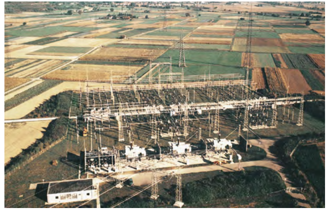
Fig. 3.1-2: Air-insulated outdoor switchgear
