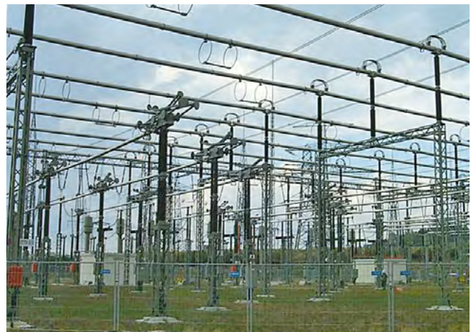
Fig. 3.1-18: Busbar disconnectors in diagonal arrangement, 380 kV, Germany
