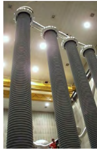
Fig. 4.2-22: Energy storage capacitor
