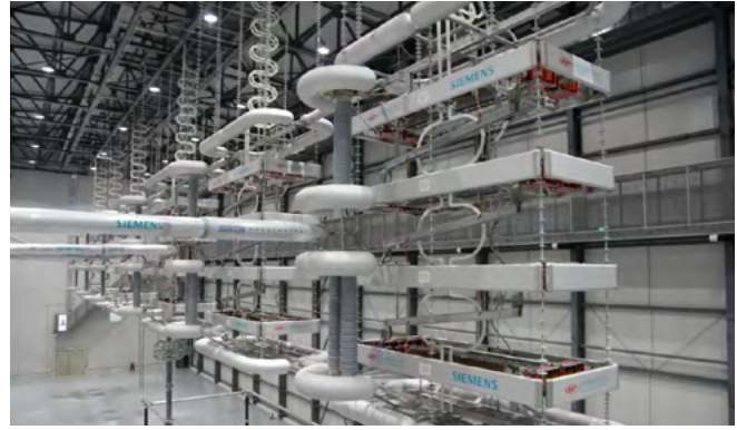
Fig. 2.2-5: UH voltage and power electronics – the thyristor valves are designed to operate at 800 kV voltage level. Yunnan-Guangdong, China
