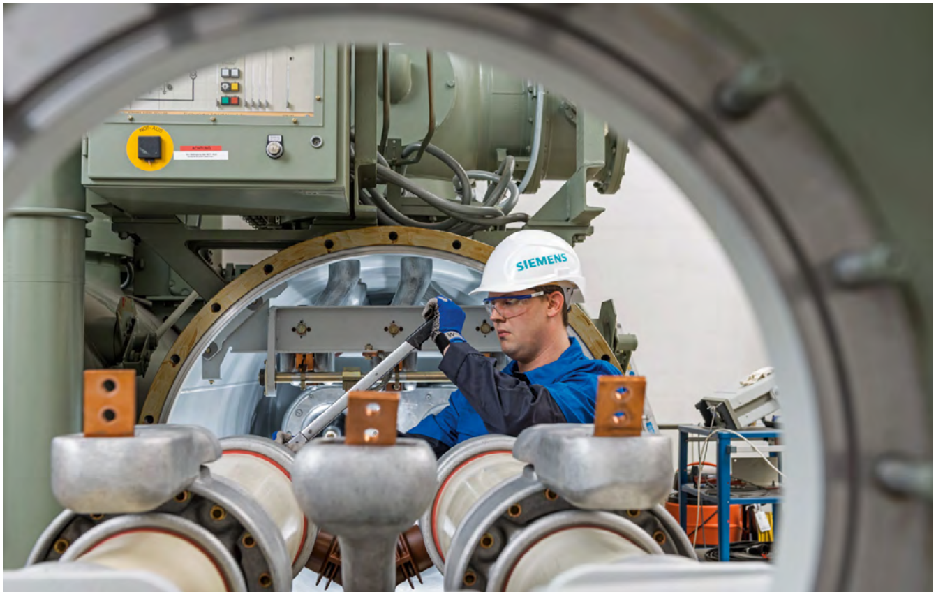
Fig. 10.3-2: Maintenance works on a HV GIS 8DN8
