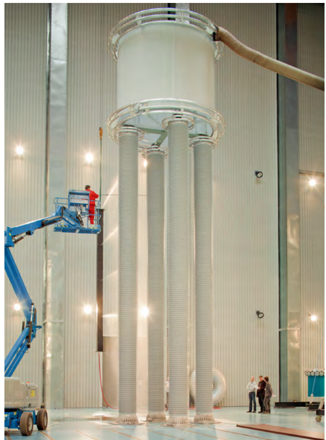
Fig. 4.2-36: Pole bus smoothing reactor for UHVDC Agra (BIL 1,300 kV; 2,680 A; 75 mH) – tests at HSP Cologne
