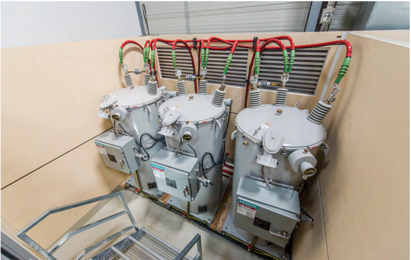
Fig. 5.11-4: In-phase voltage regulators, Niederstetten, Germany
