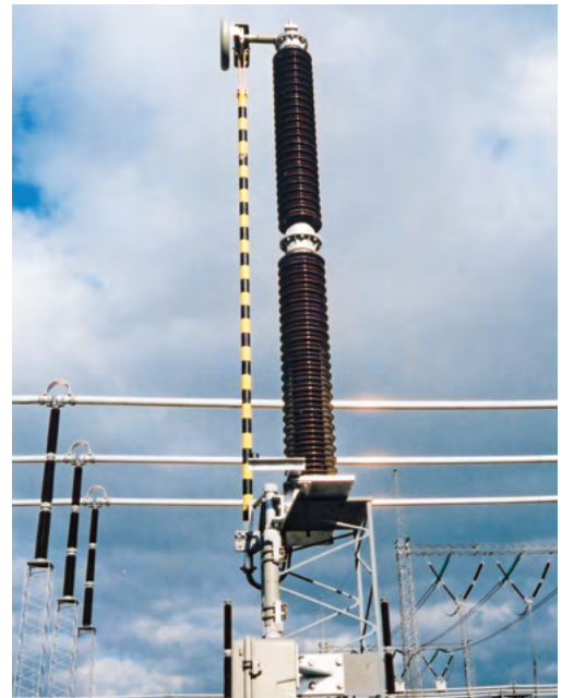
Fig. 4.1-30: Free-standing earthing switch
