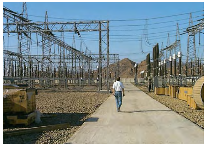
Fig. 3.1-16: Central/center tower arrangement, 220 kV, Egypt
