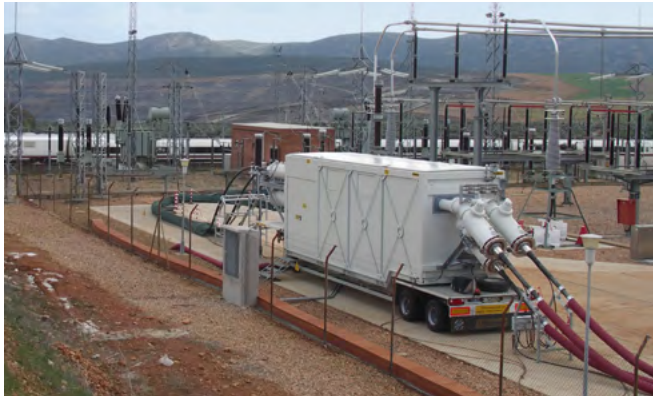
Fig. 2.4-13: 245kV Mobile substations with HV cable connection
