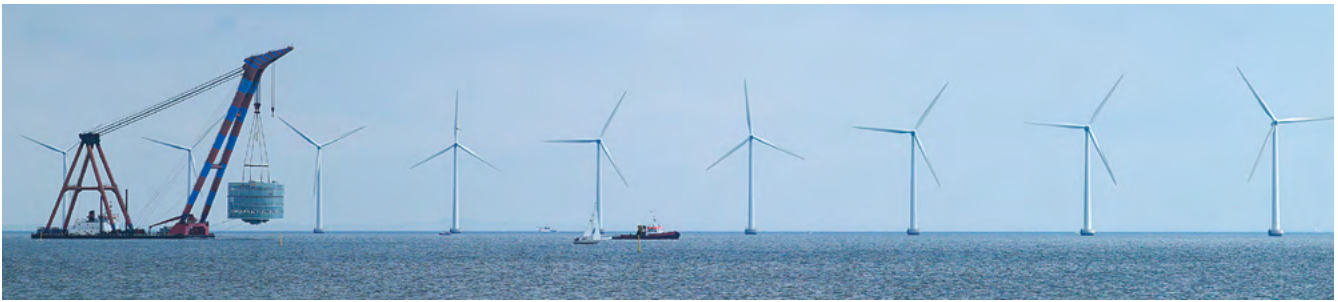
Fig. 2.2-28: Siemens executes projects as an EPC contractor
