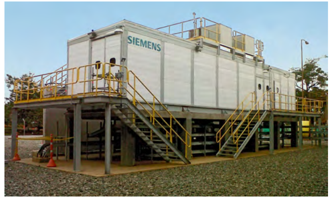
Fig. 2.4-6: E-house for mining in Columbia
