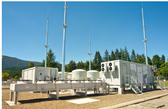
Fig. 2.2-20: SVC PLUS units in New Zealand
