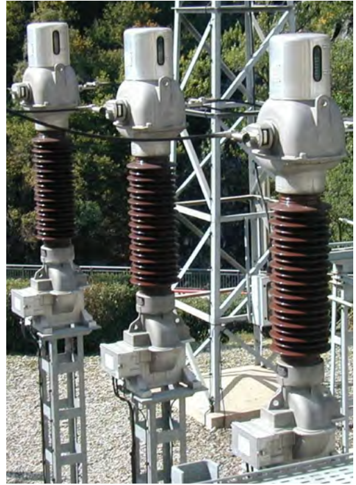
Fig. 4.2-18: 145 kV oil-immersed combined instrument transformer
