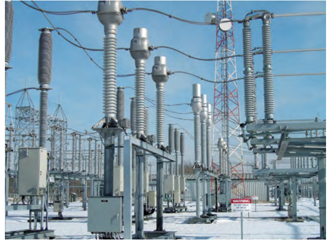
Fig. 4.2-15: 300 kV oil-immersed current transformers in Alberta, Canada
