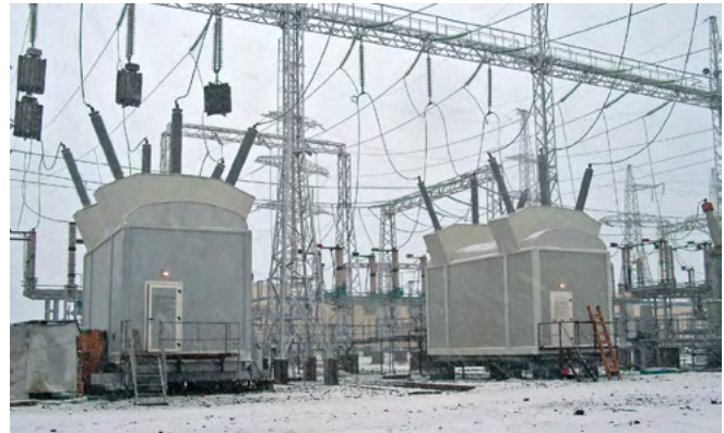
Fig. 2.4-7: 245kV E-house for Transmission utility in Siberia
