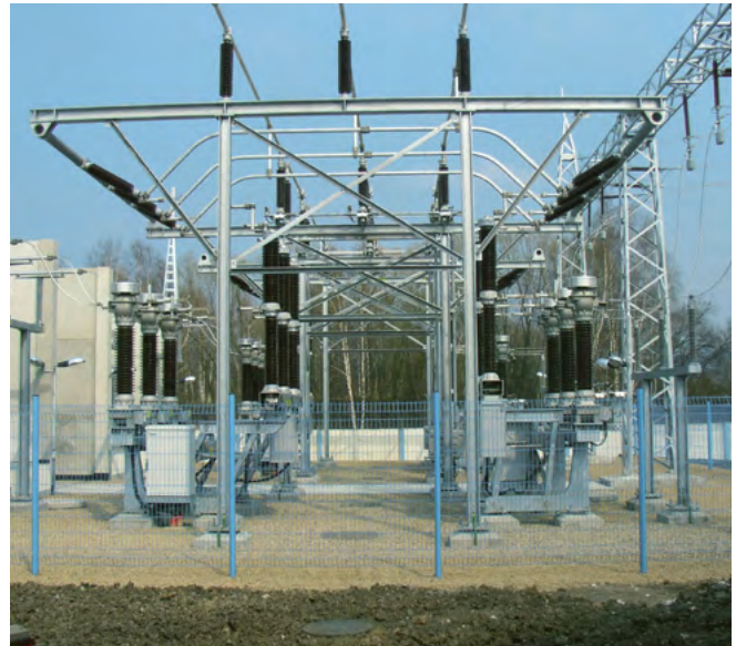
Fig. 3.1-26: H-arrangement with SIMOVER, 145 kV, Czech Republic
