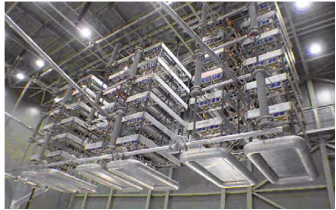
Fig. 2.2-2: Earthquake-proof and fire-retardant thyristor valves in 500 kV long-distance transmission in Guizho-Guangdong, China
