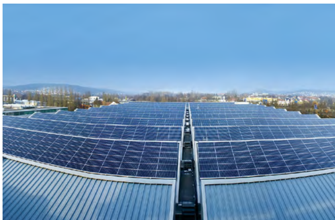
Fig. 2.3-1: SIESTORAGE offers solutions for distribution grids with a high share of distributed renewable energy sources
