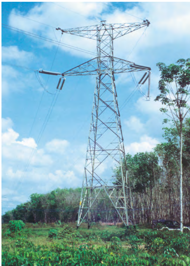
Fig. 2.2-76: 300 kV HVDC interconnector from Thailand to Malaysia (bipole transmission line)
