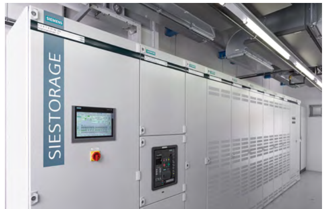
Fig. 2.3-16: SIESTORAGE system installed in an existing electrical building at the steel mill of the AMEH in Eisenhüttenstadt, Germany
