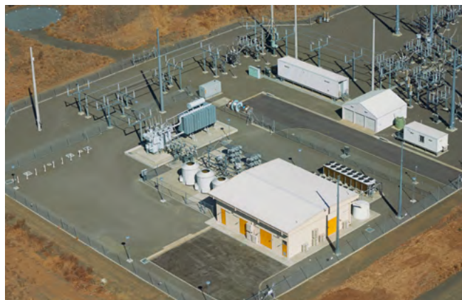
Fig. 2.2-21: Site view SVC PLUS in Australia
