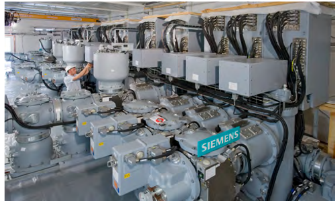
Fig. 2.4-3: High Voltage GIS E-house project for a mine, New Caledonia
