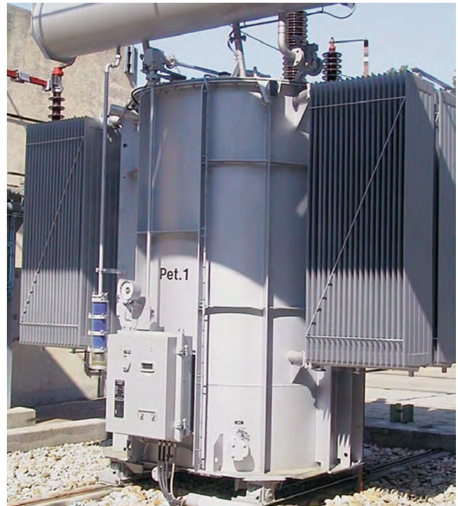
Fig. 4.2-37: Arc-suppression coil 110 kV
