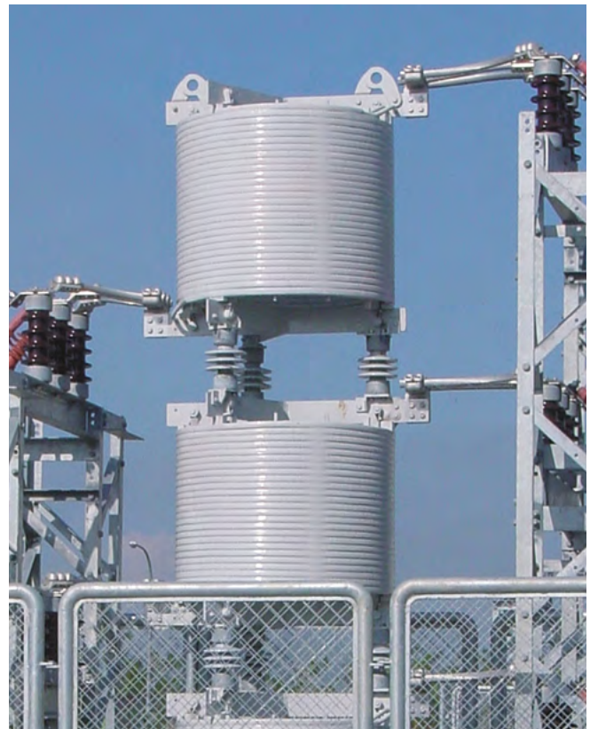
Fig. 4.2-34: 3-phase stacked current-limiting reactor
