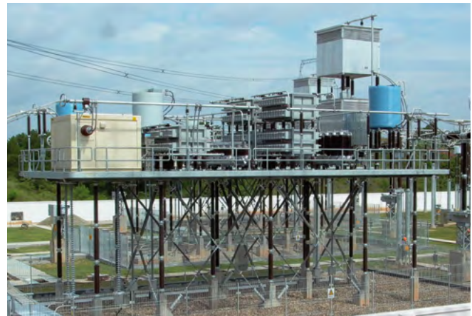
Fig. 2.2-22: View of a TCSC system
