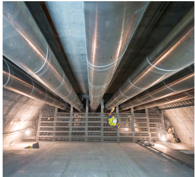
Fig. 2.2-51: Vertically installed GIL in Xiluodu, China
