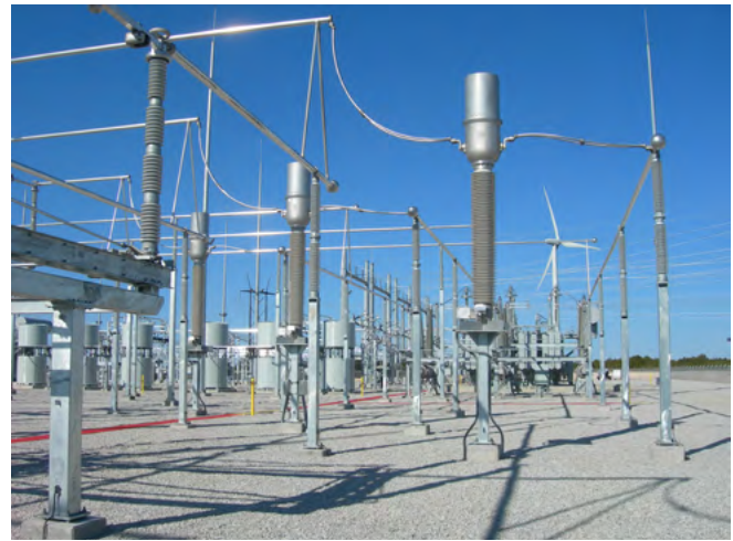
Fig. 4.2-21: 362 kV gas-filled combined instrument transformer
