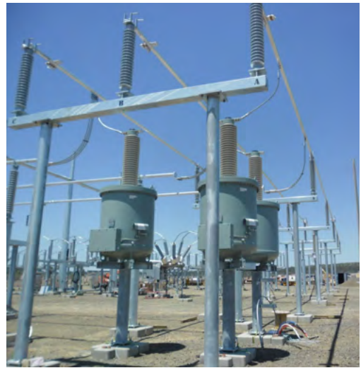
Fig. 4.2-29: 145 kV power VT for AIS
