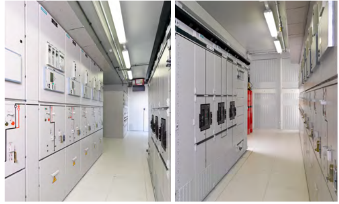
Fig. 2.4-1: E-house Project Nacala (South Africa)
