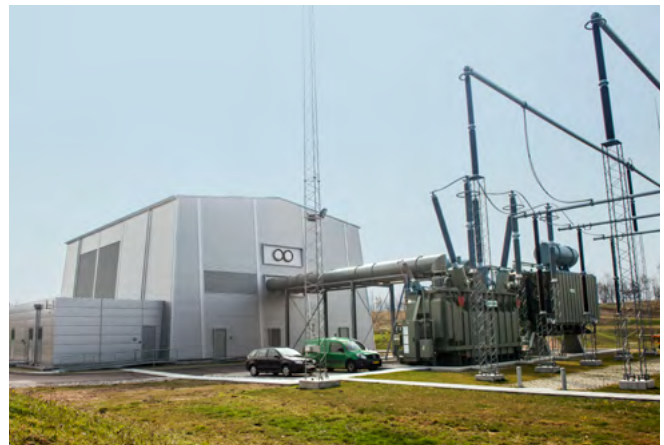
Fig. 2.2-25: Synchronous condenser in Bjaeverskov, Denmark
