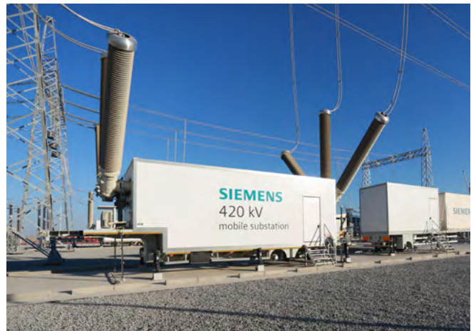
Fig. 2.4-24: world first 420kV mobile substation
