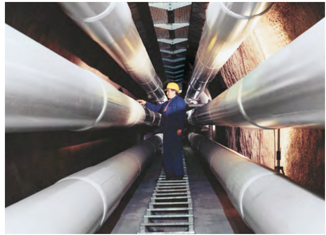
Fig. 2.2-39: GIL arrangement in the tunnel of the pumped-storage power plant in Wehr, Southern Germany (4,000 m length; in service since 1975)
