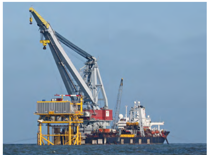
Fig. 2.2-32: 2009 300 MW Offshore Wind Farm Thanet, UK
