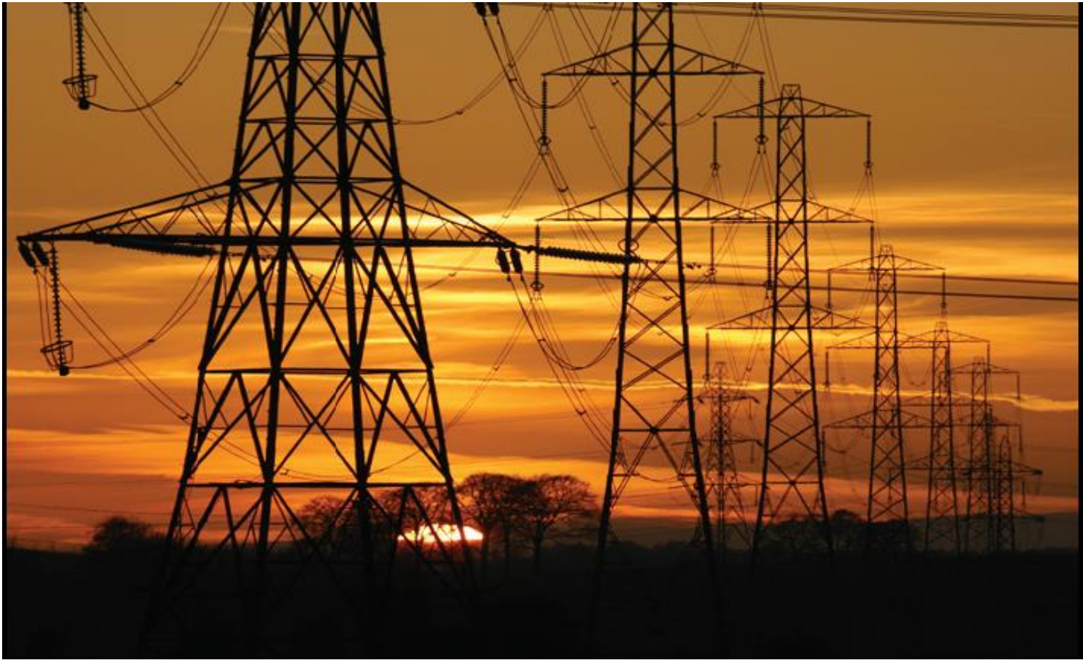
Towers showing line sag
